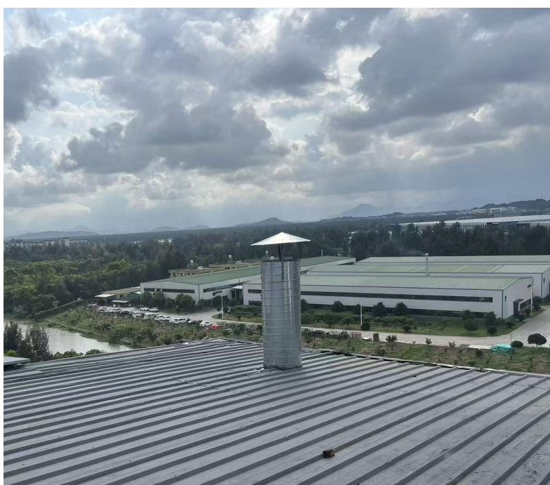
DA002 光固化涂料喷漆废气排气筒
